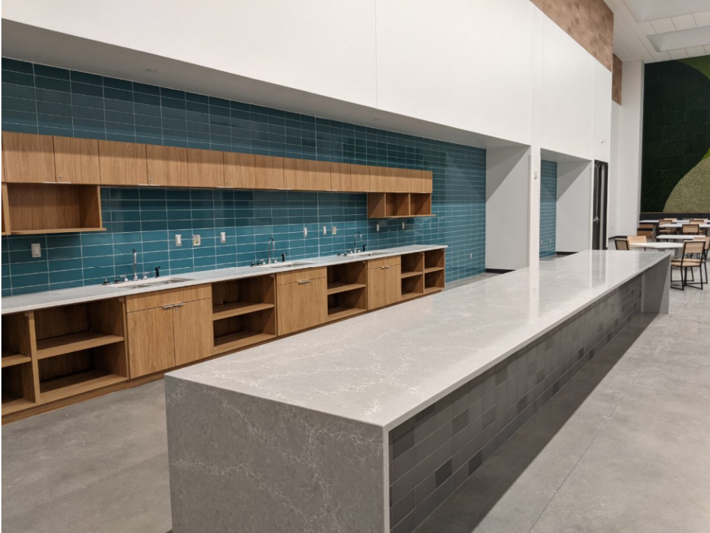
Complete installation of wall tile, cafeteria cabinets and countertops in the cafeteria/lounge area
