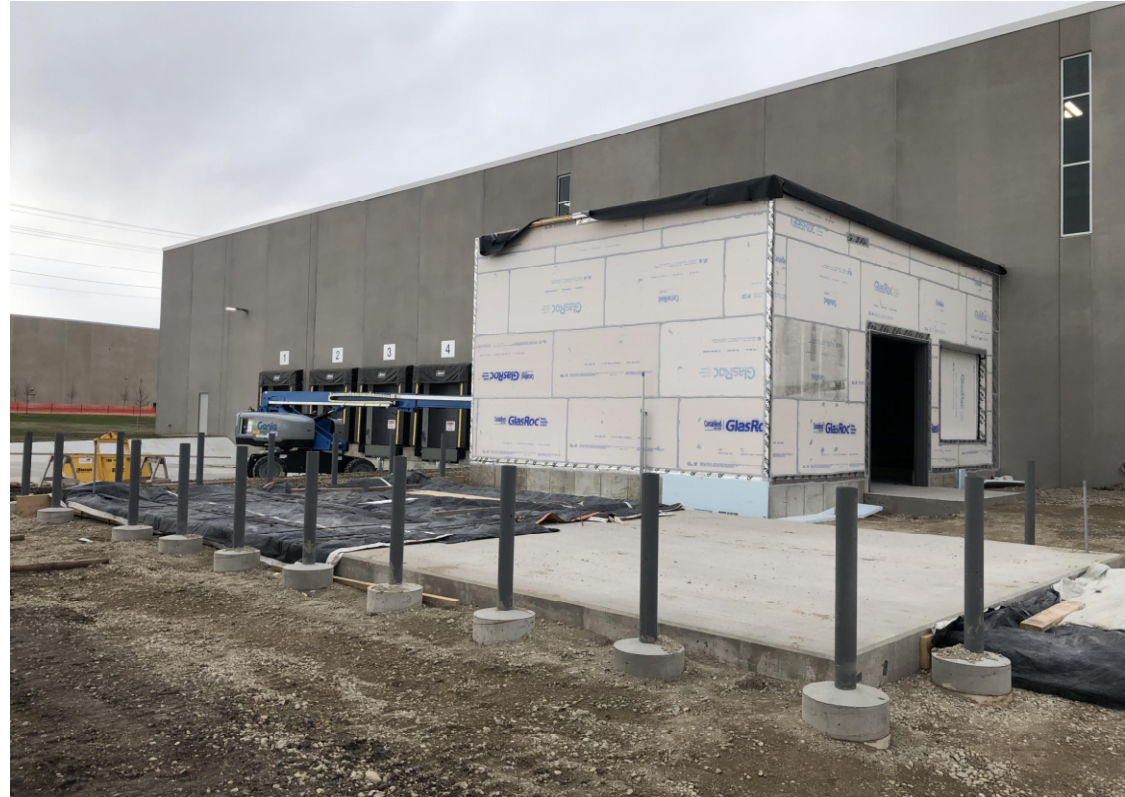
Construction begins on bump out building and is moving towards completion in December
