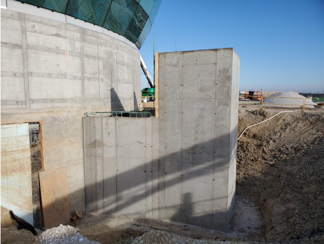
Southeast Area Well
